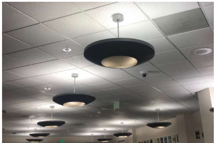
Figure 4.16: Acoustic ceiling tiles example.
