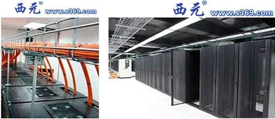
Fig. 2.67 Ceiling-mounted cabling channels
