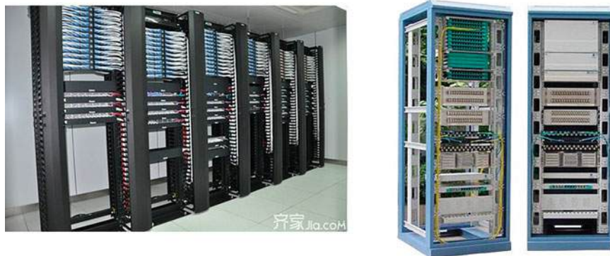
Fig. 2.8 Cable distribution cabinet in common use
