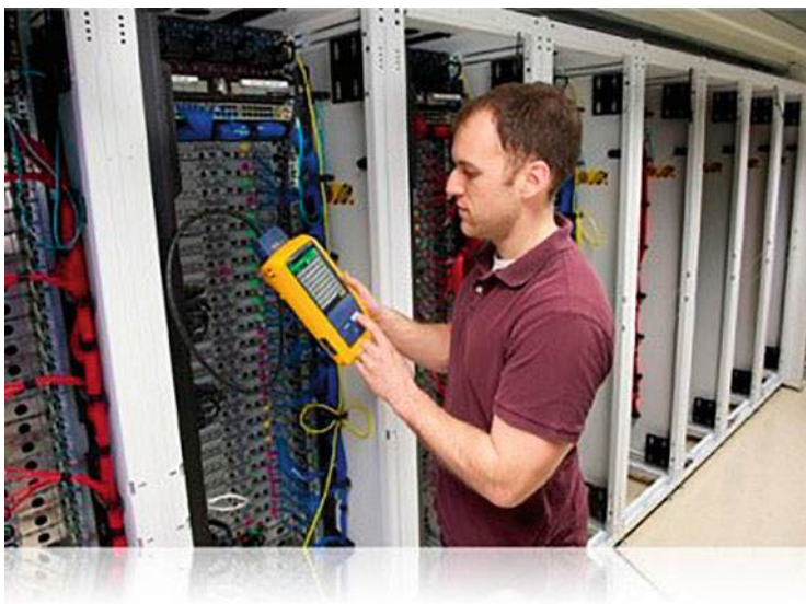
Fig. 2.51 Troubleshooting using a network tester
