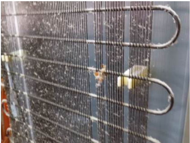
Figure 10. Typical fouling in a condenser.
